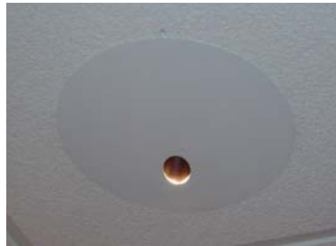
Overlapping cover plate installed in drop ceiling.
